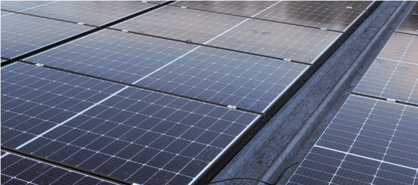
Solar panels at Eurofragrance manufacturing plant, Rubí, Spain
